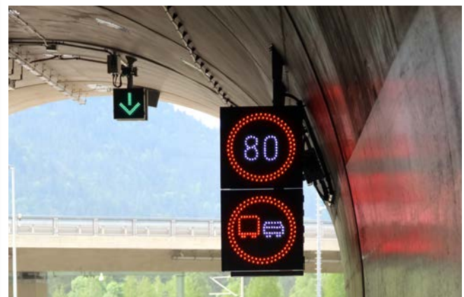
Plug connections for the continuous light signs allow quick exchange in an emergency.
