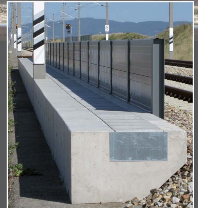
Noise Breaker after installation
